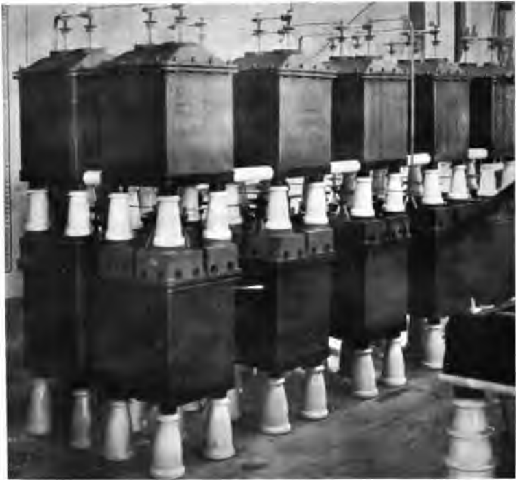
FIG. 151.—Condenser battery (Nauen).
